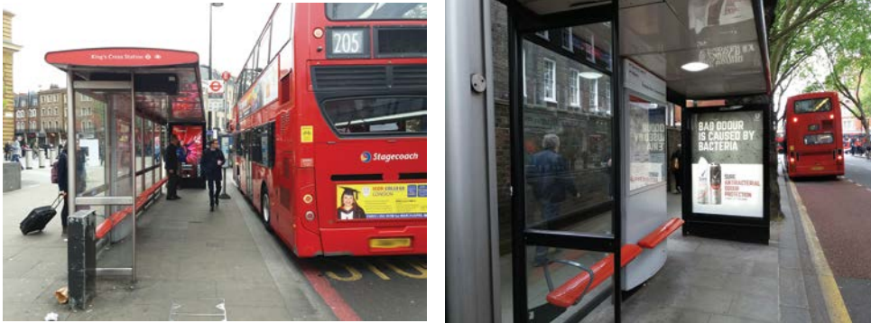
▼ Figure 7.2 Adjacent supply pillar (L) and integral electrical housing (R)
