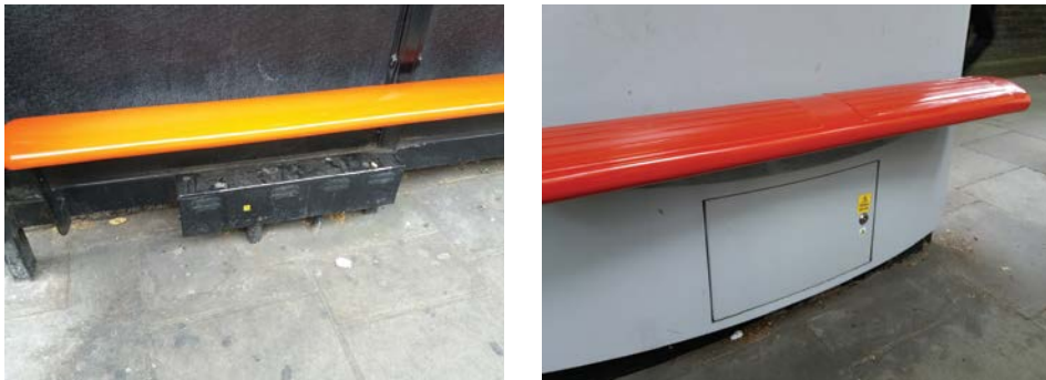
▼ Figure 7.3 Inadequate electrical compartment (L) and adequate electrical compartment (R)
