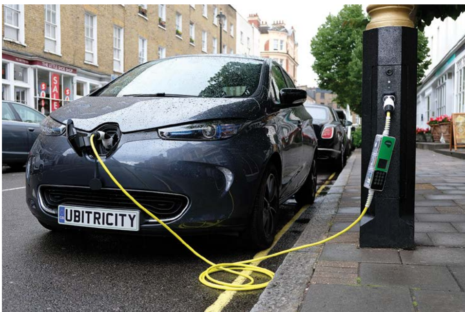
▼ Figure 5.6 Charge point integrated onto the column door (courtesy of Ubitricity)
