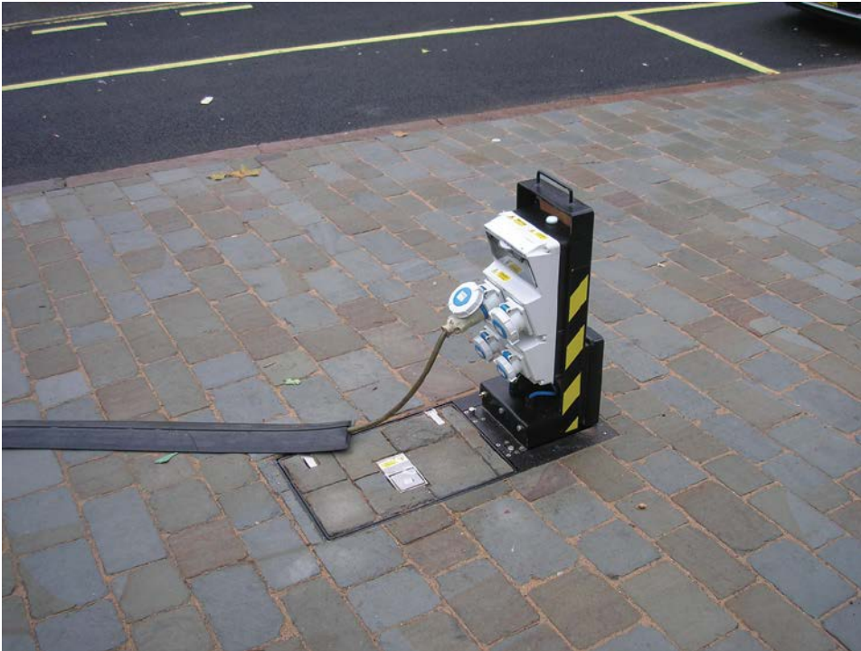
▼ Figure 6.5 Cable protection ramps
