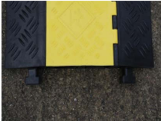
▼ Figure 6.11 Cable containment
