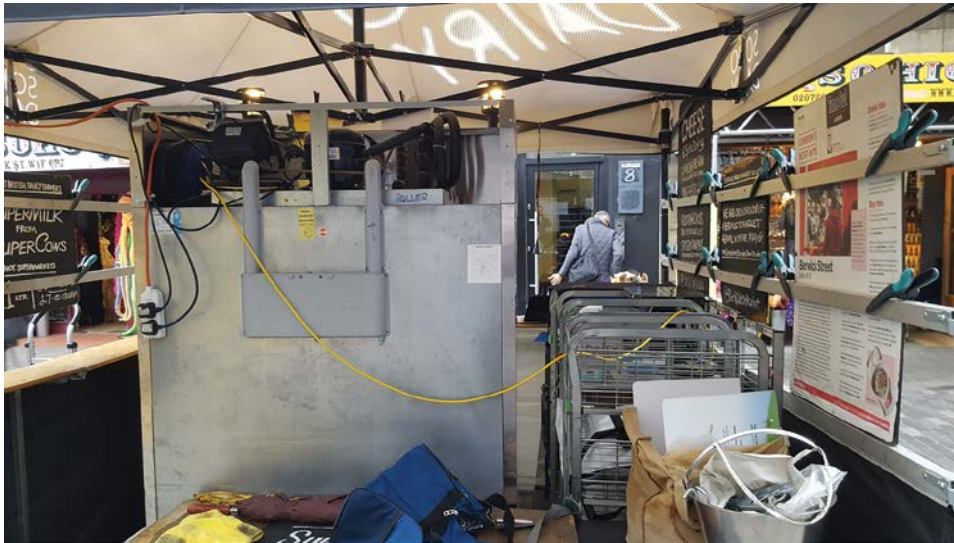
▼ Figure 6.6 Market stall with multiple extension leads and incorrectly terminated cables
